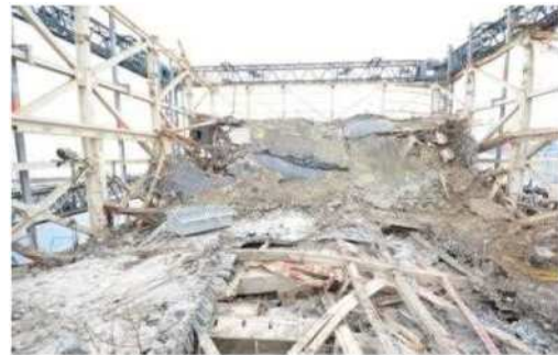
Condition of the collapsed south-side roof
